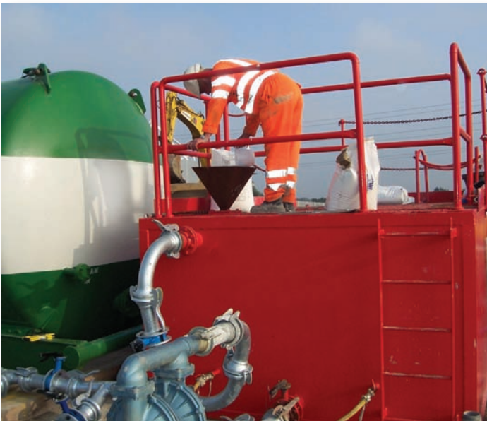
Mixing in Surface Tanks
